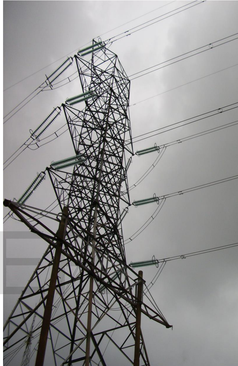
Figure 7: Twin line 330kv running from National Grid/ Delta 1
