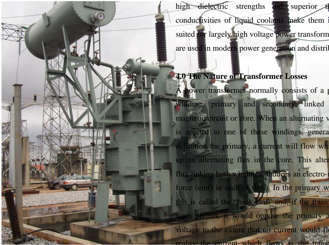
Figure 4: 60MVA 132KV / 33KV Power Transformer
